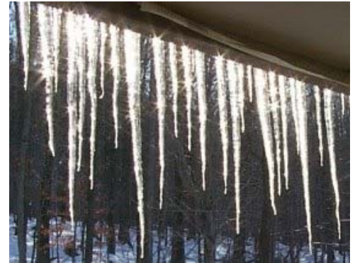
Abundant icicles mean you may be at risk for water damage due to ice dams
